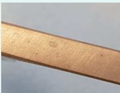
Fig. 3: Example of minor corrosion
